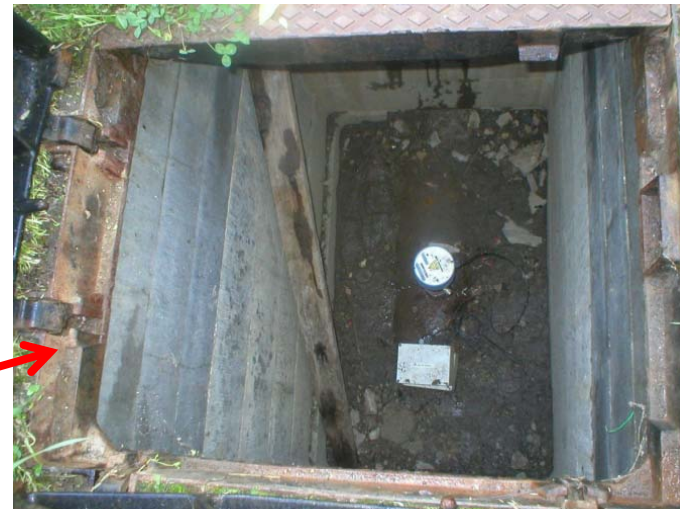
A water pipe inside a manhole. There may be some wireless sensors to measure water flow and pressure.
